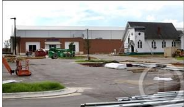
The parking lot on the southeast side of the Rocky Mount Event Center is lined with construction equipment and materials on Aug. 22 in downtown Rocky Mount.
